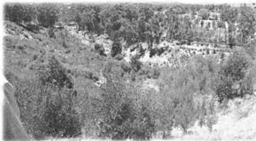
Figure 5: the vegetation encroaching the dam wall of Idas Valley Dam 2.
